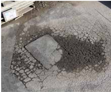
A typical "alligator skin" asphalt failure
