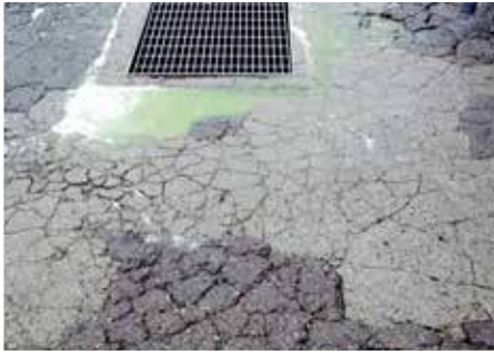
A typical "alligator skin" asphalt failure.
