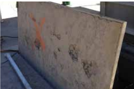
Failed overlay product on a municipal utility access door
